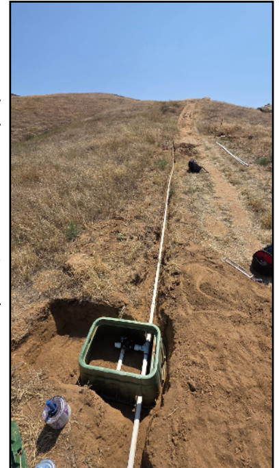
Mainline and valves
