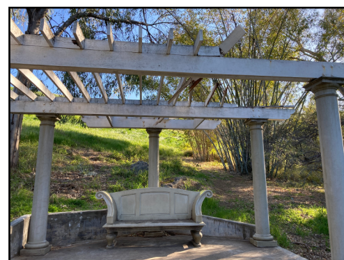
Damage on the Celebration of Life Memorial
