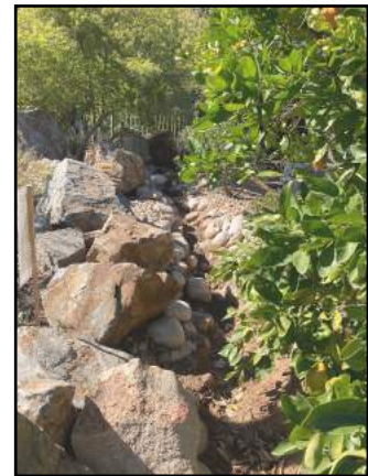
Butterfly Garden drainage channel
